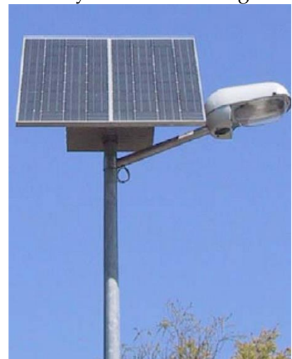
Figure: Solar Powered Street Light
